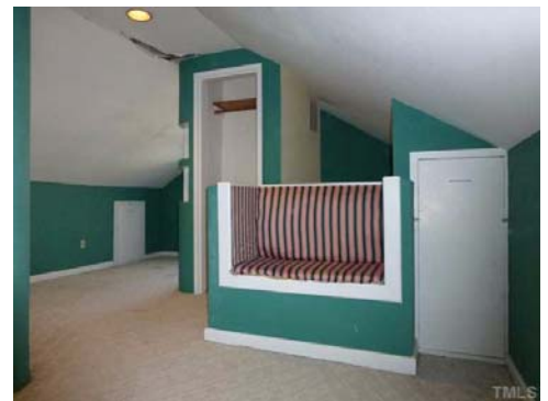
The loft is divided into two spaces by a full bath. The exploratory hole in the ceiling was again made by Steve Smallman who found no leaks.
