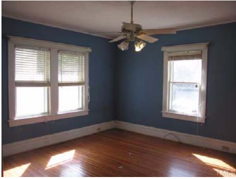
In the back bedroom, Steve Smallman opened the ceiling to check out an earlier leak that now appears inactive. He also determined that the wall crack is due to termite damage visible in the basement. The owners are selling as-is.
