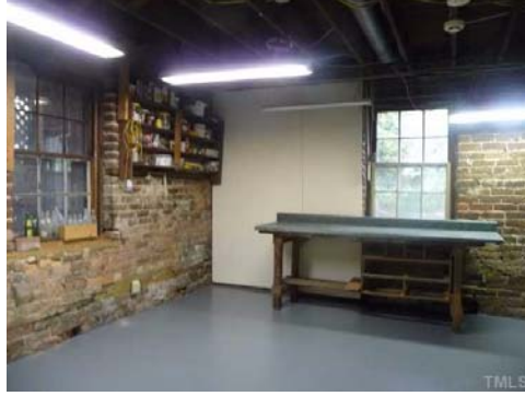
Workshop, studio, storage, whatever - this is one of the two unfinished lower level spaces. The other includes the furnace and additional flexible space.
