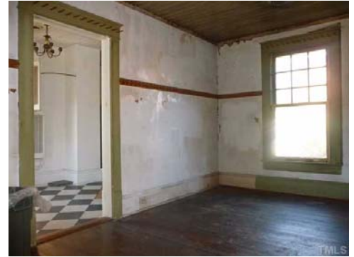
Ok, we said it needs work. This is the back bedroom looking into the laundry room that can also be a closet for the bedroom. Not shown is the wall where plaster had been removed as part its earlier use as a workshop. <BR/>
