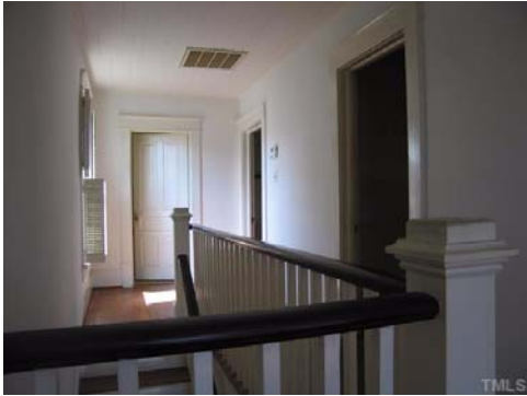
Upstairs again, the hall leads past the three bedrooms to a full bath. There are options for adding a 2nd upstairs bath to create a true master suite. A floor plan is available.
