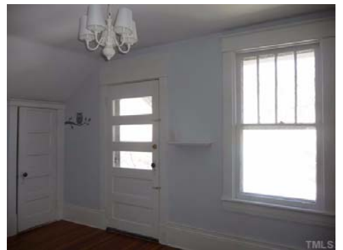
The second upstairs bedroom includes a door leading to exterior metal stairs that once provided access to an upstairs apartment. The stairs could easily be removed and sold for scrap.
